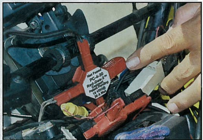
Photo D—Anderson Power Pole connectors make for easy power hookups and—with the plugs used as a standard by club members—easy swapping of radios as well.
